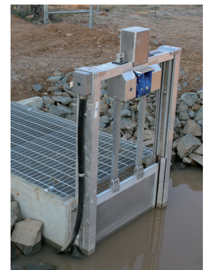
Electronic flow meter with the control gate on the farm side of the outlet
