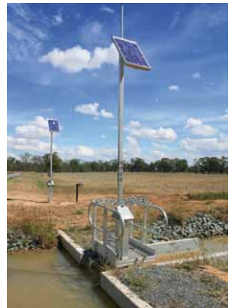
Foreground: FlumeGate™ meter Background: 375 mm Magflow meter
