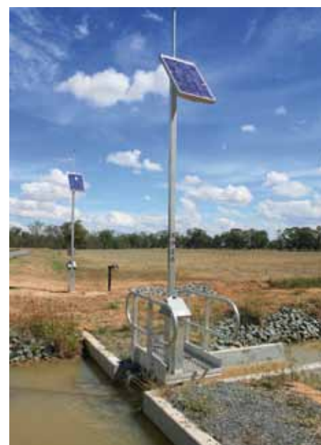
Foreground: FlumeGate™ meter Background: 375 mm Magflow meter
