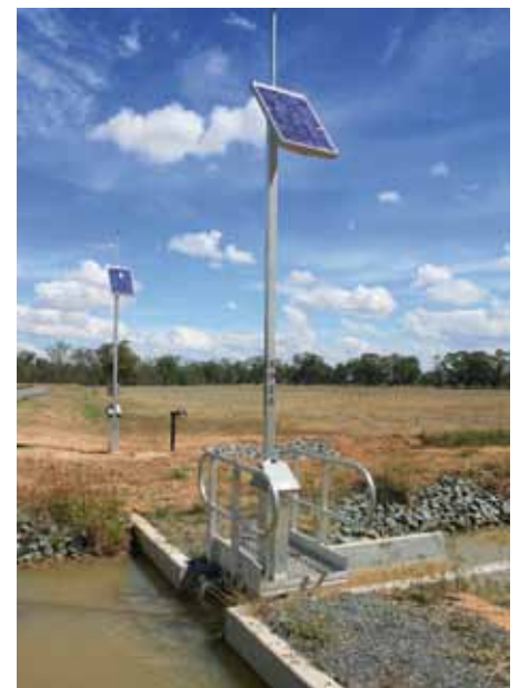
Foreground: FlumeGate™ meter Background: 375 mm Magflow meter
