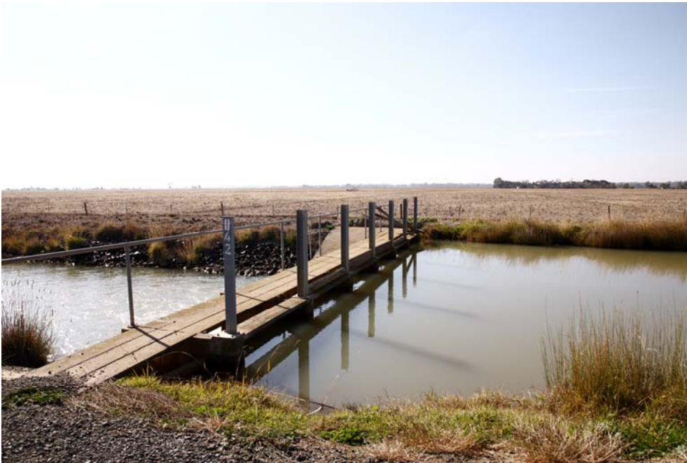
Figure 1: Gates on a channel before automation
