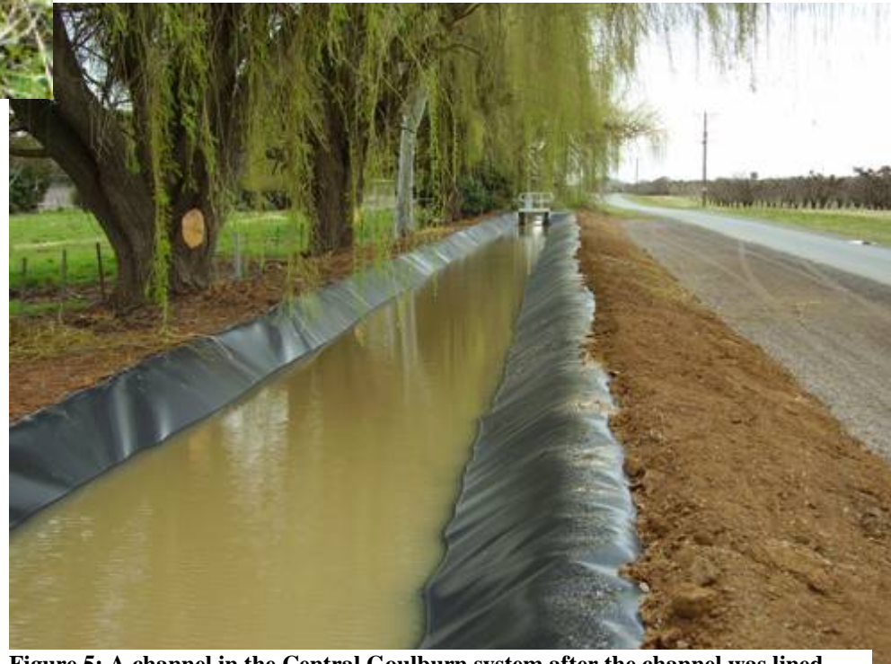
Figure 5: A channel in the Central Goulburn system after the channel was lined with HDPE plastic.
